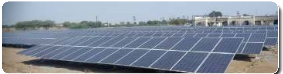
657kWp Ground Mounted SPV Power Plant installed at Nimboni, Solapur (Maharashtra) under EESL Project
